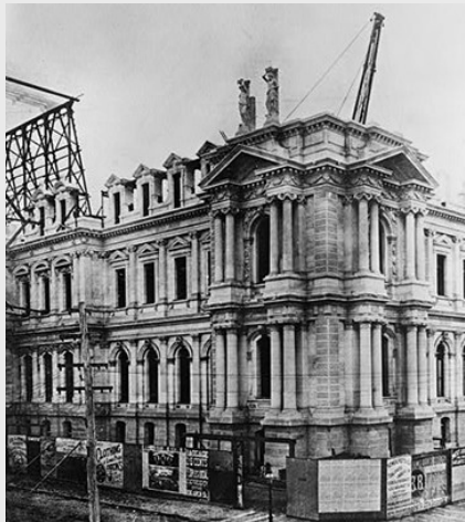
City Hall, Philadelphia, PA. Southeast Pavillion Under Construction, 1881. Historic American Buildings Survey.
